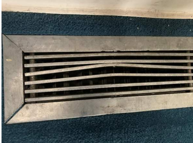
Photo 15: Existing damaged floor diffuser
