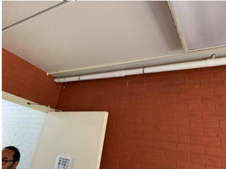
Photo 36: exposed piping in O'Connor dormitory entry
