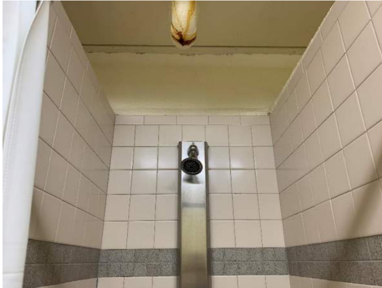
Photo 57: typical institutional type shower fixture with concealed piping cover
