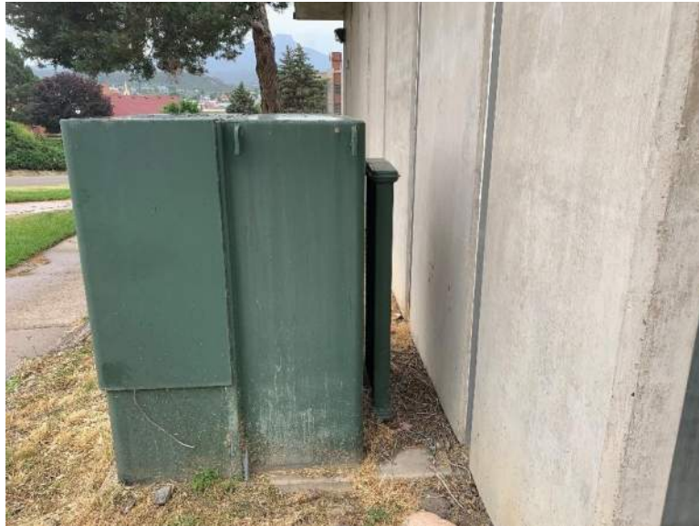
Photo 2: 75 kVA service transformer
