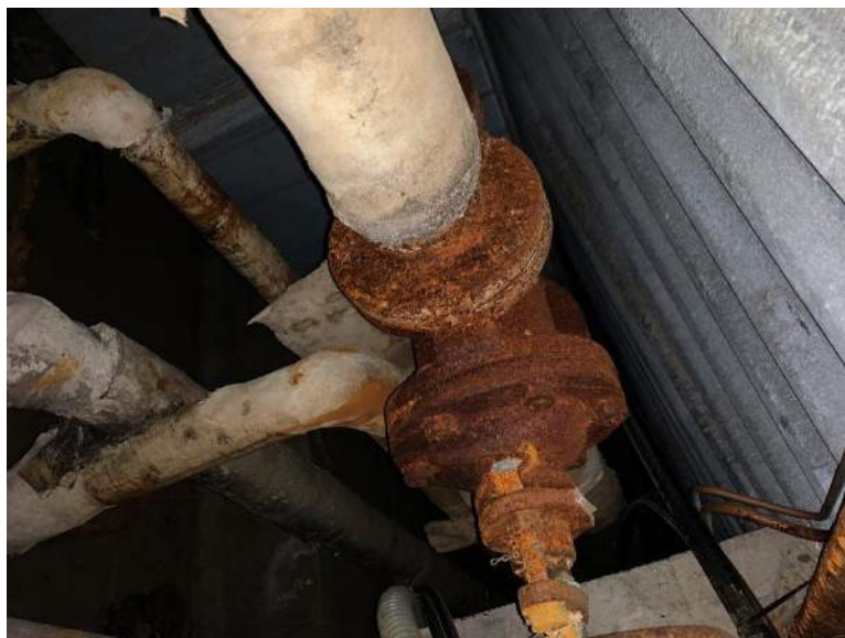
Photo 9: existing gate valve exhibiting extreme corrosion
