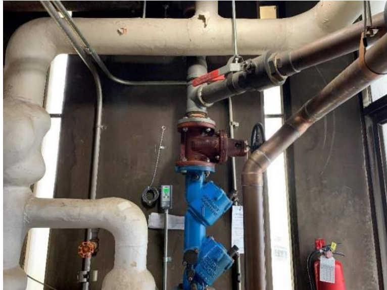
Photo 7: Domestic service water entrance
