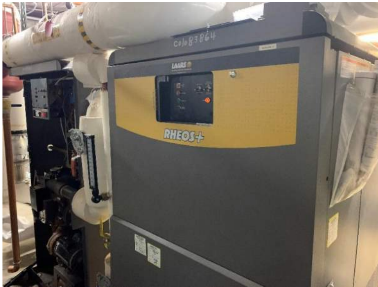
Photo 60: 2009 condensing boiler replacement
