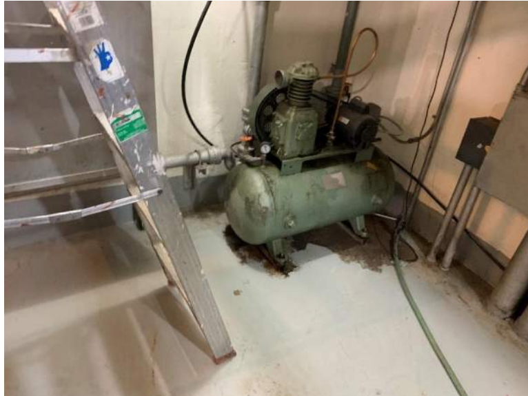
Photo 45: O'Connor pneumatic control air compressor
