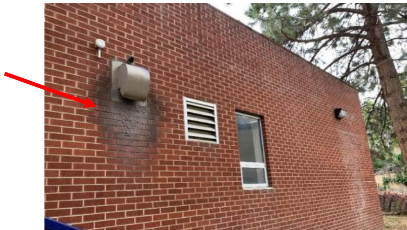
Photo 62: Lint accumulation at dryer vent
