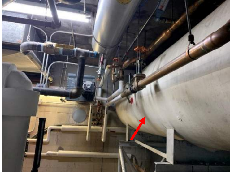
Photo 63: Existing original Huggins Hall domestic water storage tank
