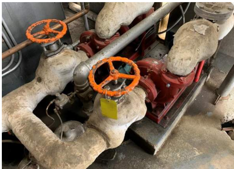
Photo 6: HW distribution pumps
