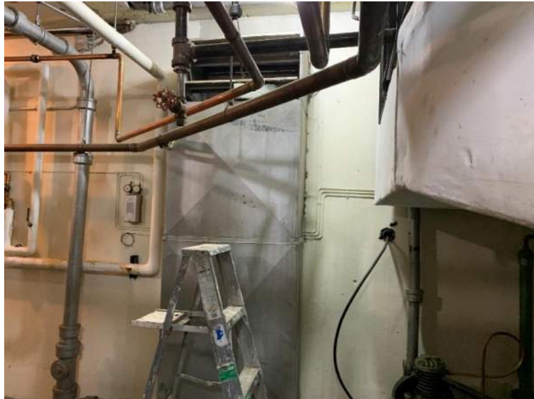
Photo 44: O'Connor combustion air ductwork
