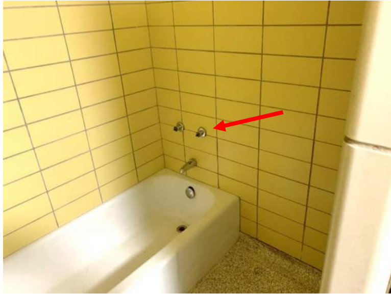
Photo 25: Existing bathtub with valve control removed?
