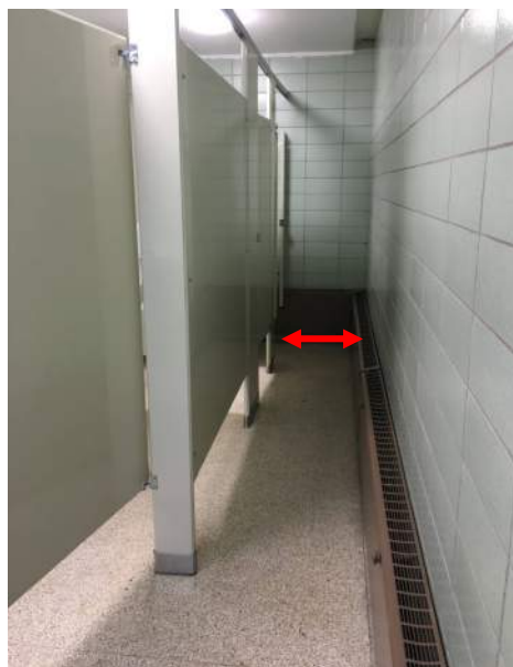
Figure J. Width of a standard aisle in a public bathroom measures 19" with convactor. Current code minimum is 36". Source: Hall Architects
