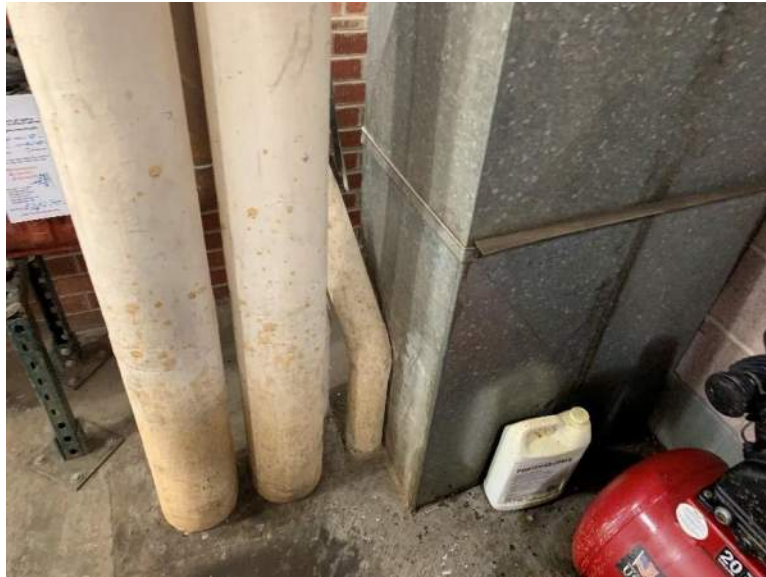
Photo 8: piping and ductwork to tunnel system
