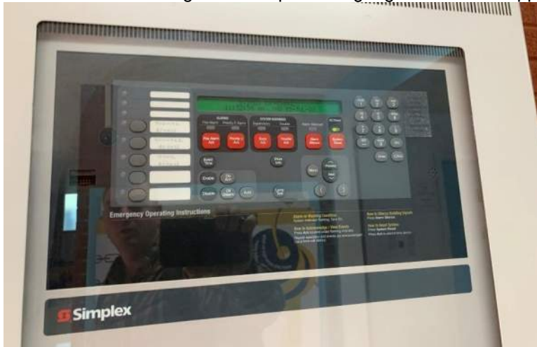
Photo 50: Huggins fire alarm system
