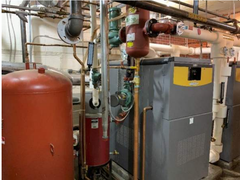
Photo 40: O'Connor Dorm replacement boilers (Laars model no. not legible on photo) installed approximately 2009
