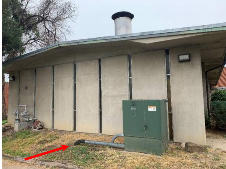
Photo 1: Student Center electric and gas utility services
