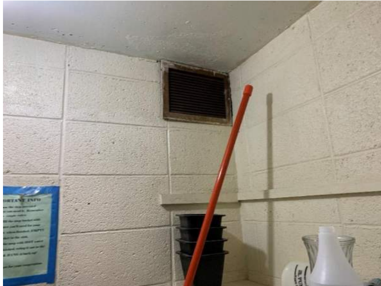
Photo 28: Johnson Residence Hall janitor closet exhaust
