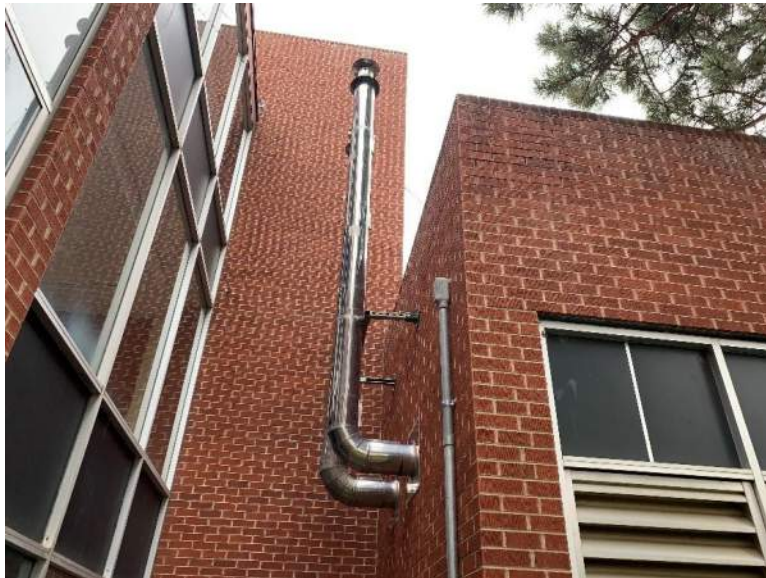
Photo 61: Category 4 Al29-4C stainless steel boiler vents
