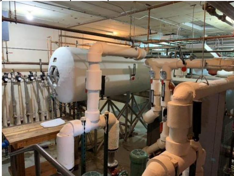
Photo 38: O'Connor boiler room with irrigation header adjacent to domestic hot water storage tank
