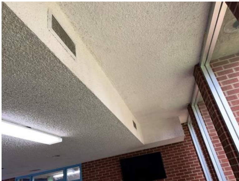
Photo 59: Bulkhead diffusers at Huggins from concealed ducted cabinet unit heaters
