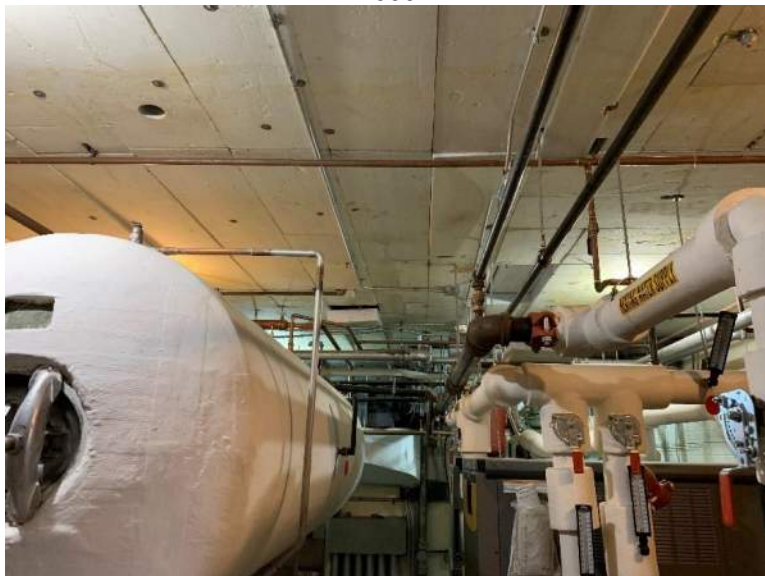
Photo 41: 1964 vintage 790 gal DHW storage tank still utilized
