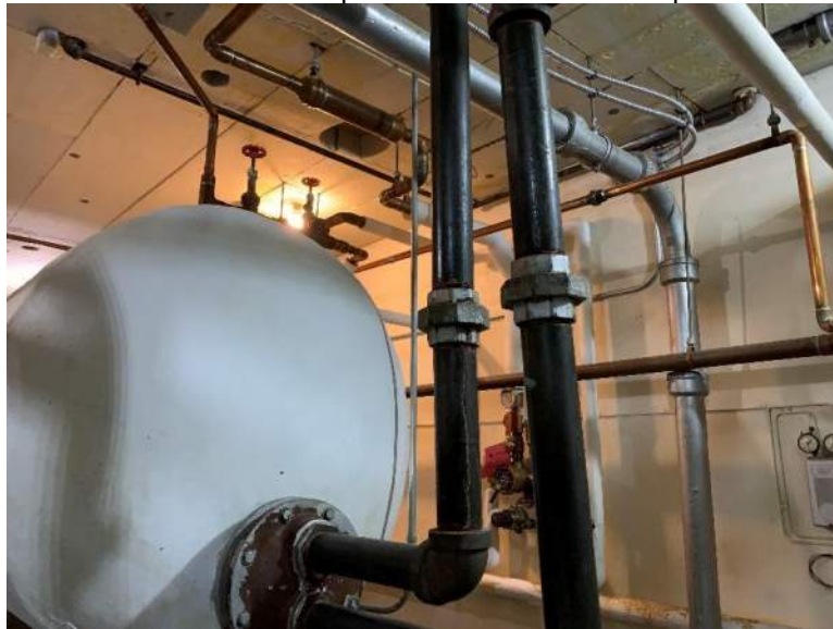
Photo 46: O'Connor domestic hot water storage tank
