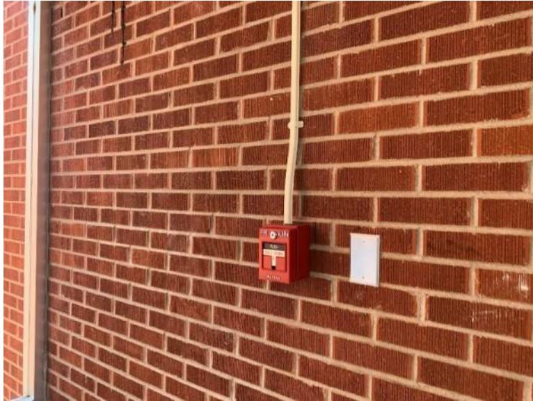
Photo 54: Typical fire alarm pull station cabled via surface mounted raceway
