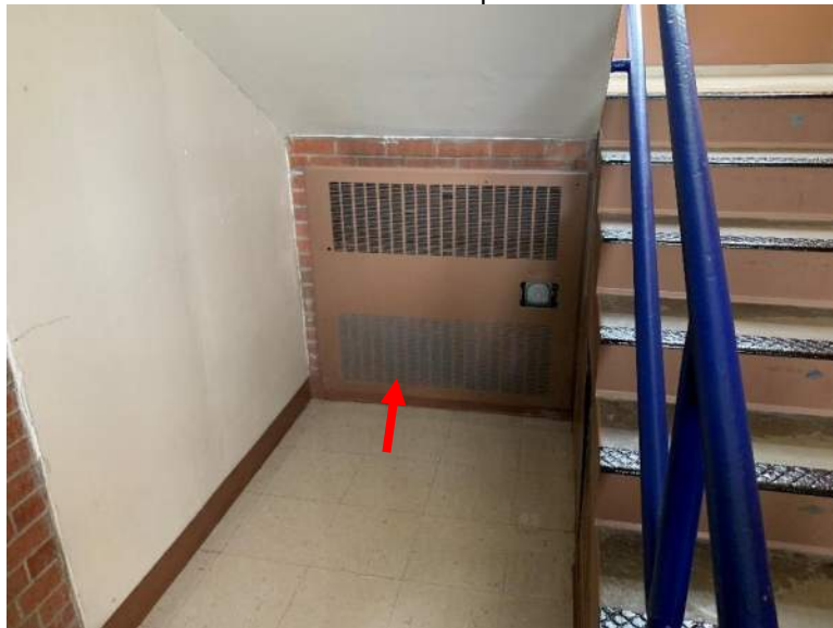
Photo 20: Johnson stairwell convection heater
