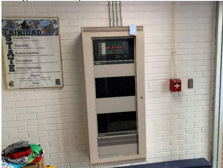
Photo 55: O'Connor Hall fire alarm control panel
