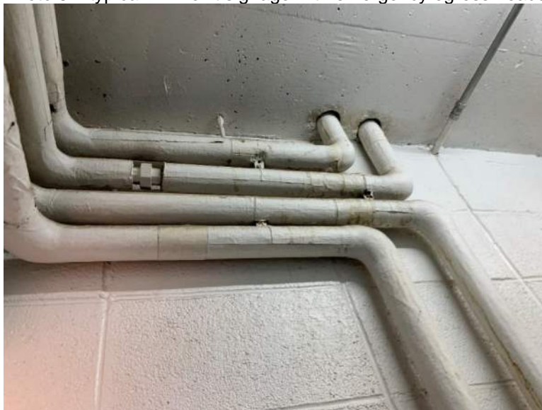
Photo 53: Suspect hard-cast ACM insulation elbows
