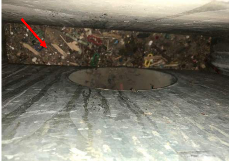
Photo 16: Existing below floor ductwork with accumulation of debris
