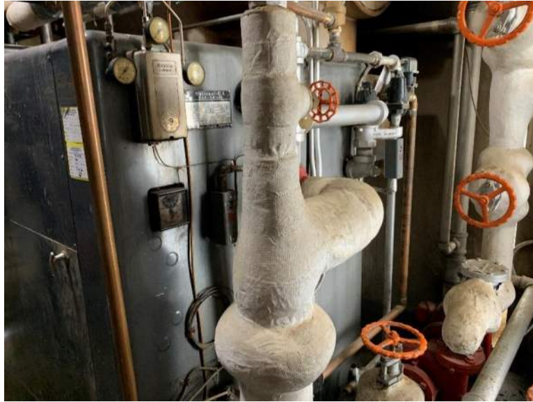
Photo 4: Existing gas-fired 3000 MBH hydronic boiler
