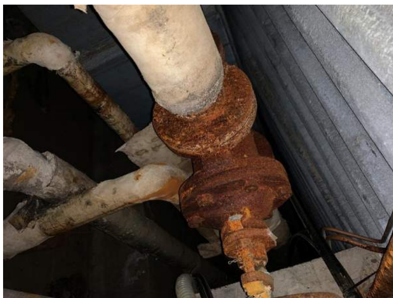
Photo 9: existing gate valve exhibiting extreme corrosion
