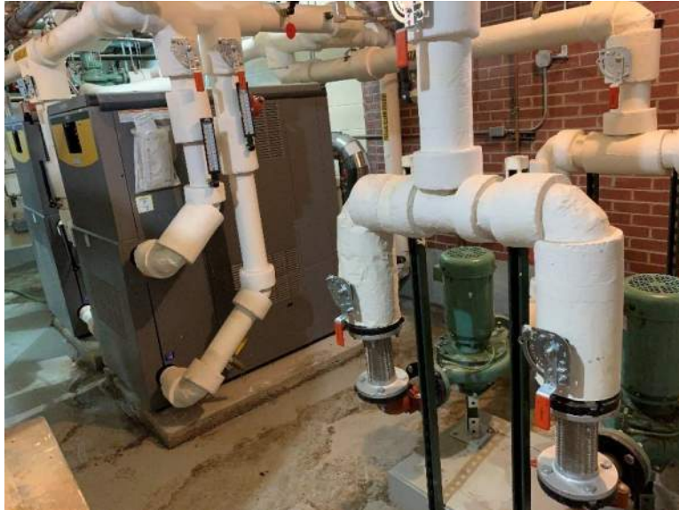
Photo 39: O'Connor boilers manufactured in August 2009 per nameplate
