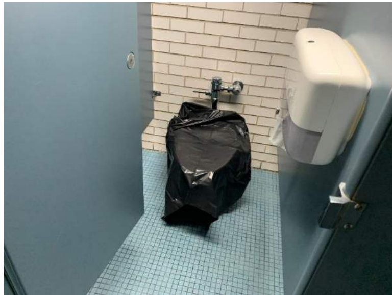
Photo 64: nonfunctional water closet
