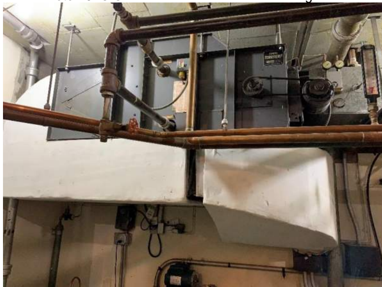
Photo 47: O'Connor heating & ventilating unit in boiler room
