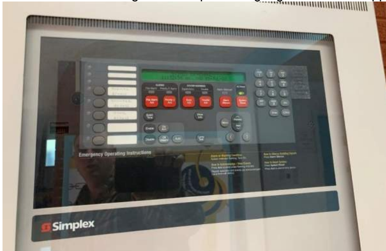
Photo 50: Huggins fire alarm system
