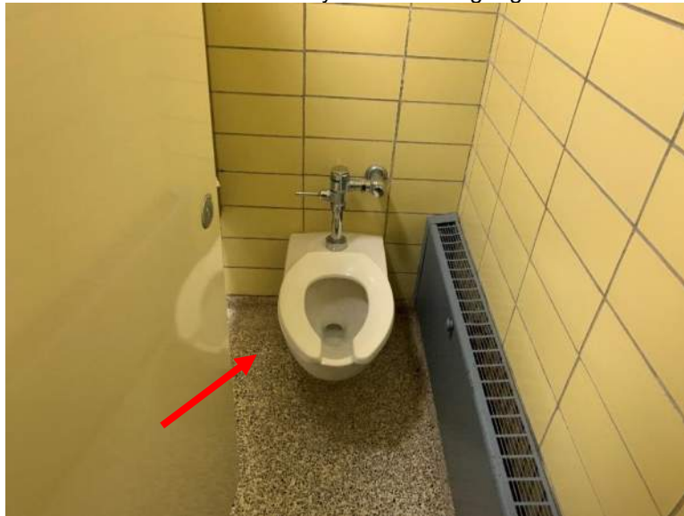
Photo 23: Existing wall-mounted American Standard 1.6 GPF flush type water closet
