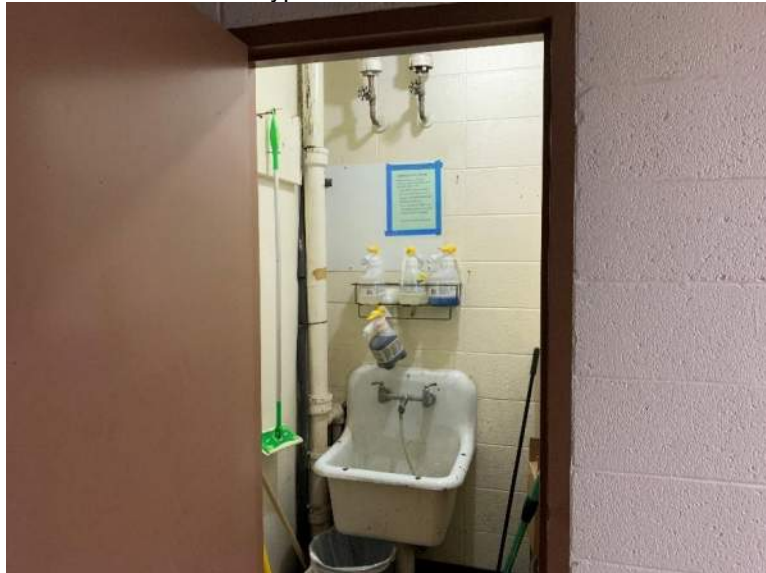
Photo 27: Johnson 3rd floor janitor sink, vent stack, and water hammer arresters
