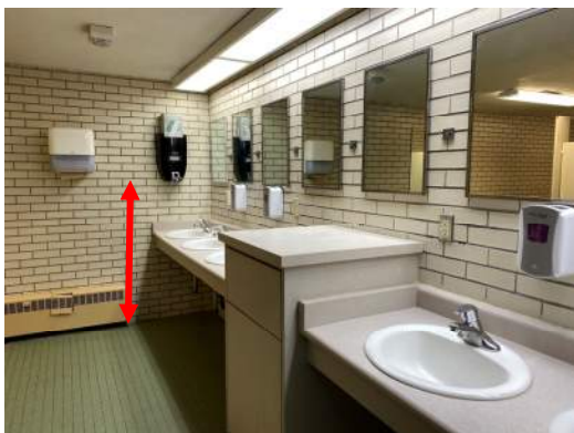
Figure K. Plastic laminate countertops appear dated, vulnerable to delamination from high moisture environments. Bottom of mirrors are set high above floor. Source: Hall Architects.
