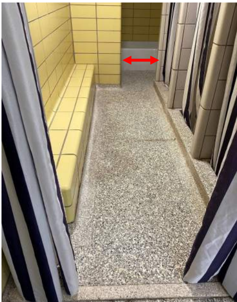
Figure I. Width of access to a public bathtub area measures 19". Current code minimum is 36". Source: Hall Architects
