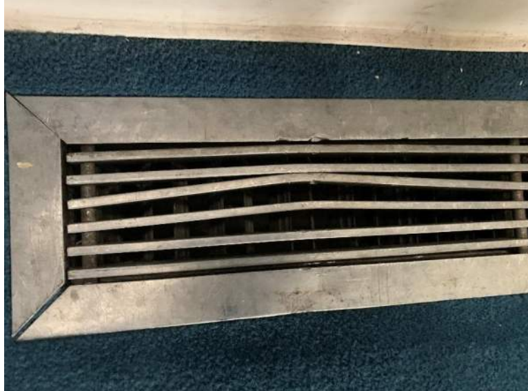
Photo 15: Existing damaged floor diffuser
