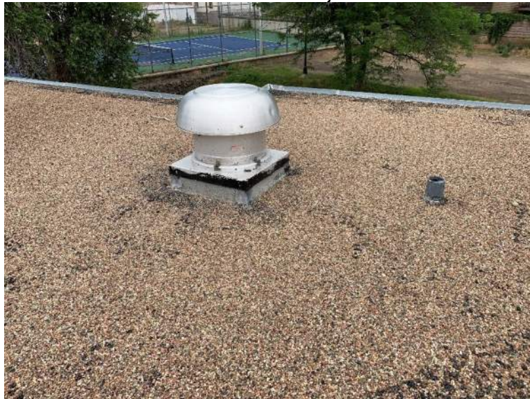
Photo 29: Johnson Dormitory Jenn-Air Model 161 HCB-A roof exhauster with 1/8 hp 115 V motor
