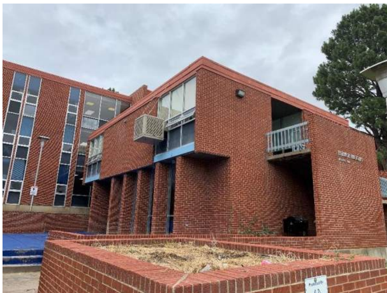
Photo 56: Huggins Hall resident apartment evaporative cooler
