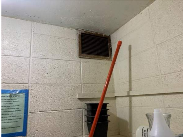
Photo 28: Johnson Residence Hall janitor closet exhaust
