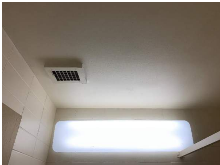
Photo 12: Women's toilet exhaust grille
