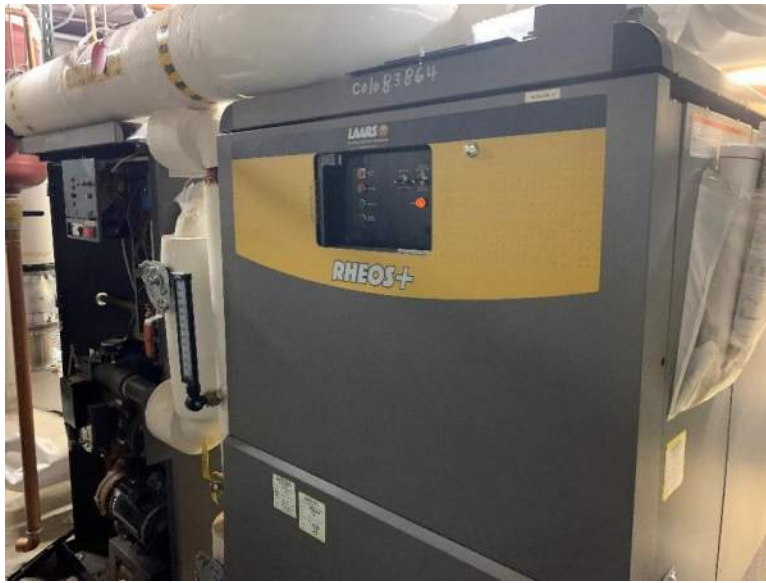
Photo 60: 2009 condensing boiler replacement
