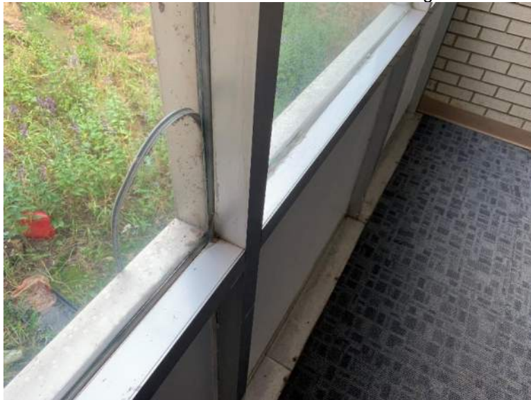
Photo 35: Single pane aluminum window with seal failure
