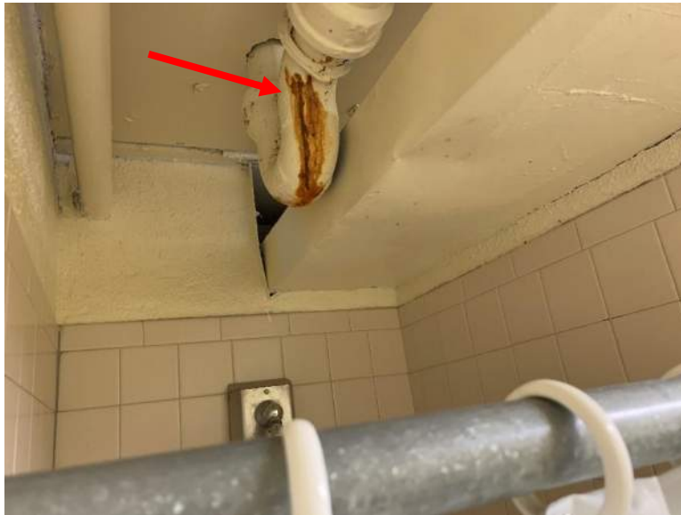
Photo 58: corrosion observed on exposed cast-iron sanitary trap
