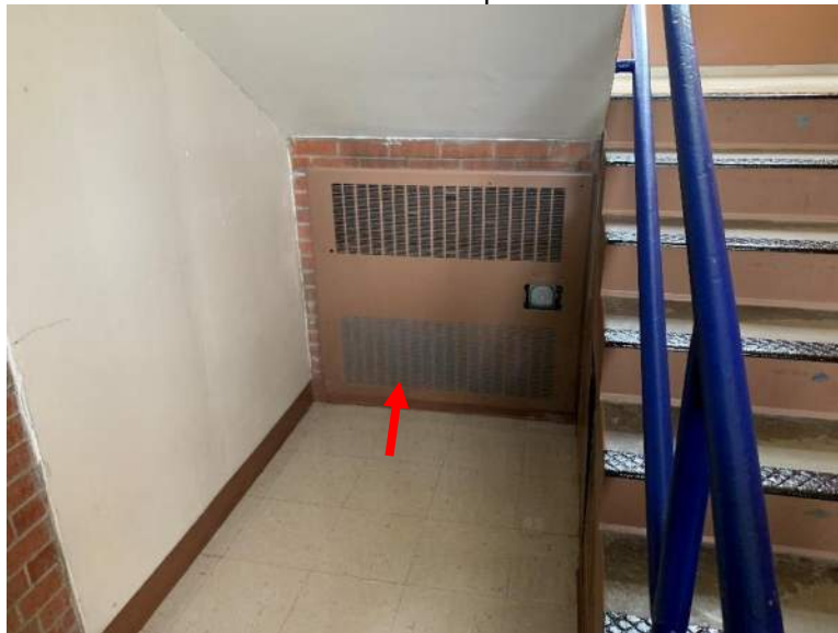
Photo 20: Johnson stairwell convection heater
