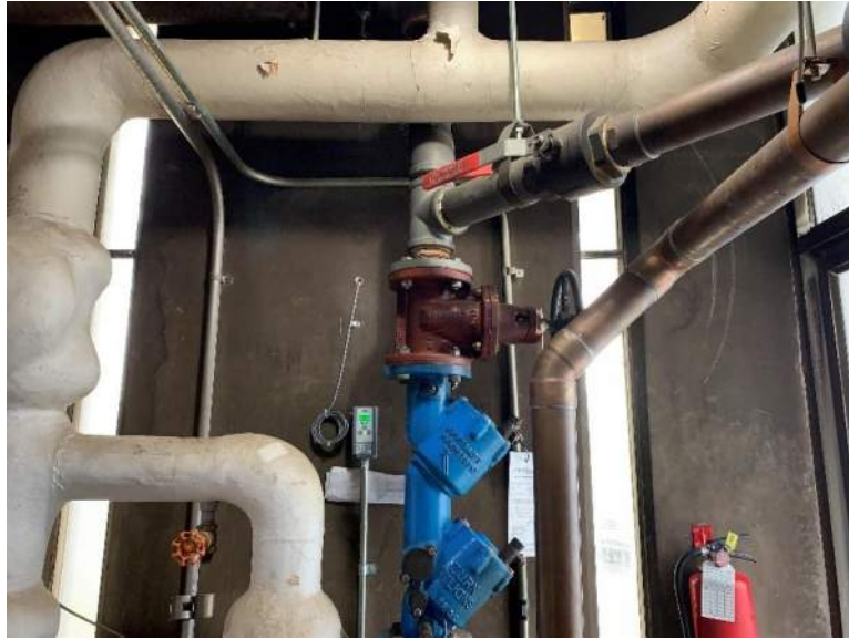
Photo 7: Domestic service water entrance
