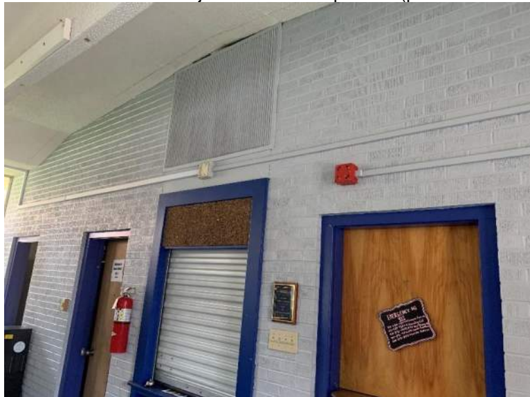
Photo 11: Return air grille for Student Center air handler unit
