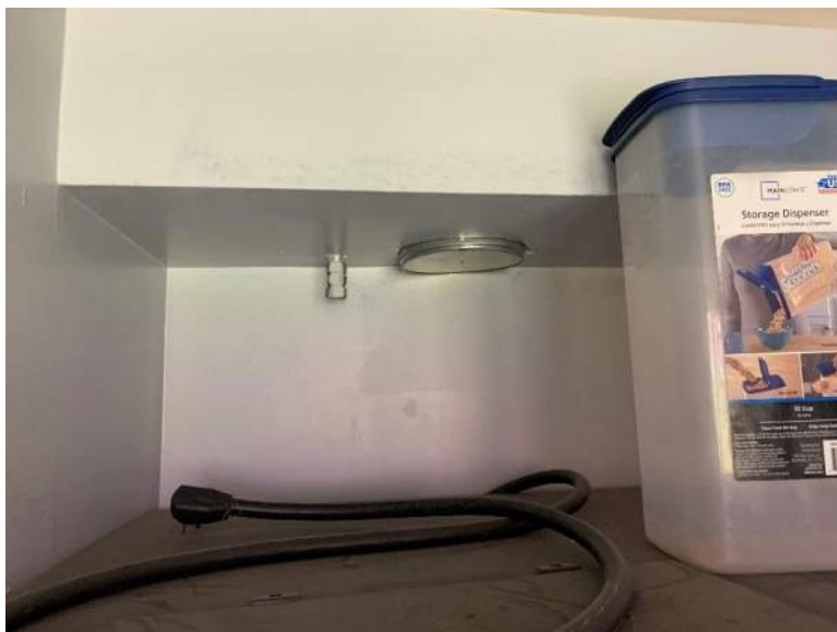
Photo 18: Abandoned duct and pipe above vending machine
