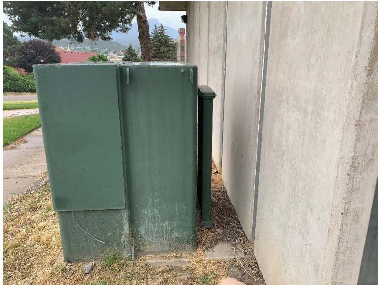
Photo 2: 75 kVA service transformer
