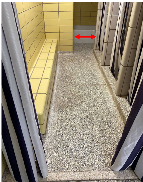
Figure I. Width of access to a public bathtub area measures 19". Current code minimum is 36". Source: Hall Architects
