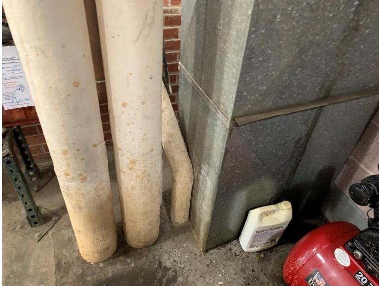
Photo 8: piping and ductwork to tunnel system
