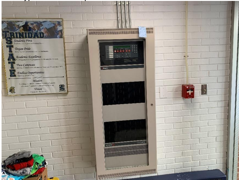
Photo 55: O'Connor Hall fire alarm control panel
