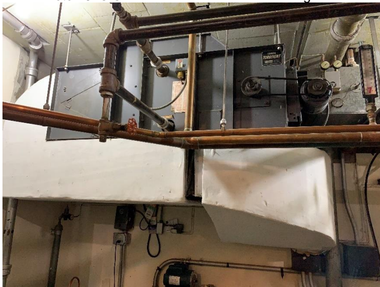
Photo 47: O'Connor heating & ventilating unit in boiler room
