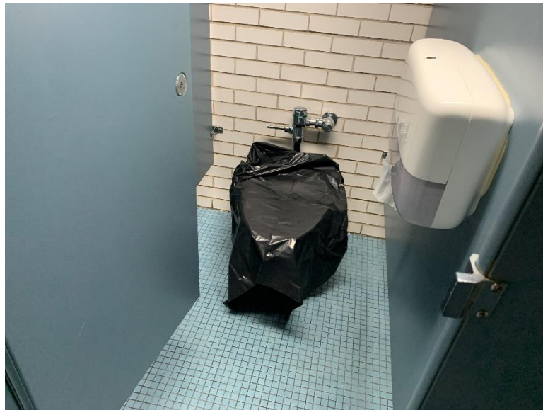
Photo 64: nonfunctional water closet
