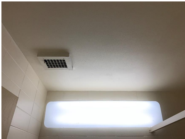
Photo 12: Women's toilet exhaust grille
