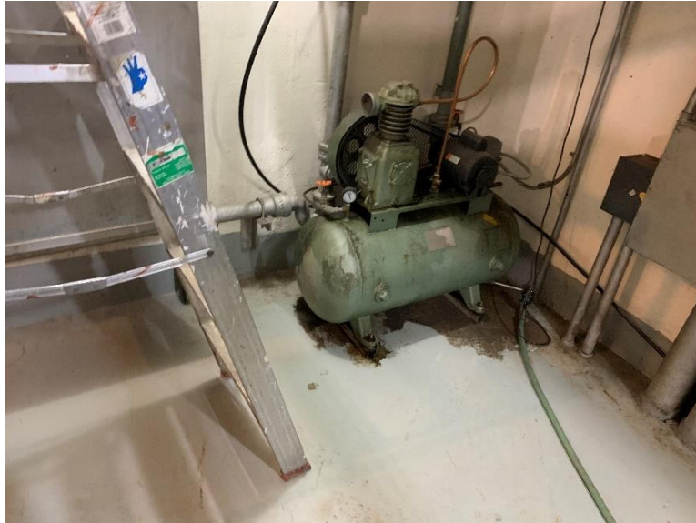
Photo 45: O'Connor pneumatic control air compressor
