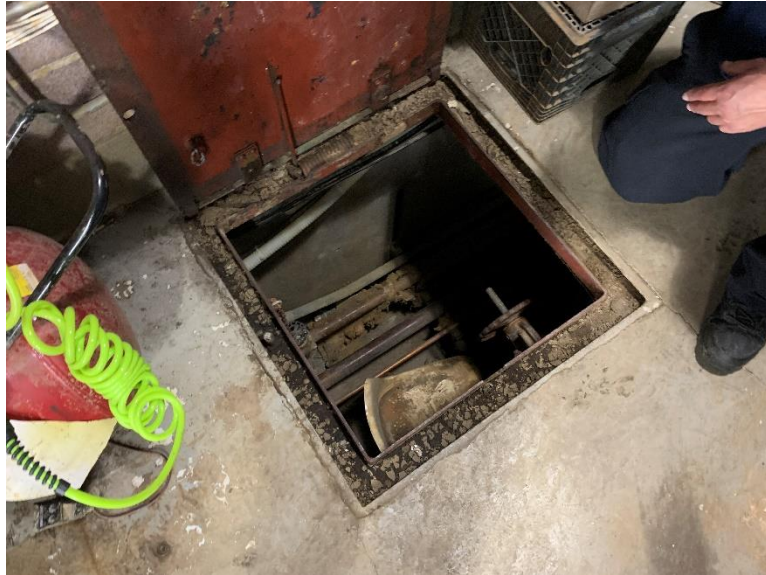
Photo 10: Tunnel access adjacent to air compressor (pneumatic control?)
