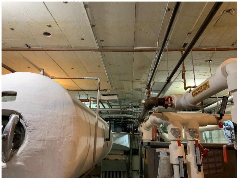
Photo 41: 1964 vintage 790 gal DHW storage tank still utilized
