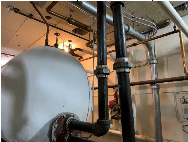
Photo 46: O'Connor domestic hot water storage tank
