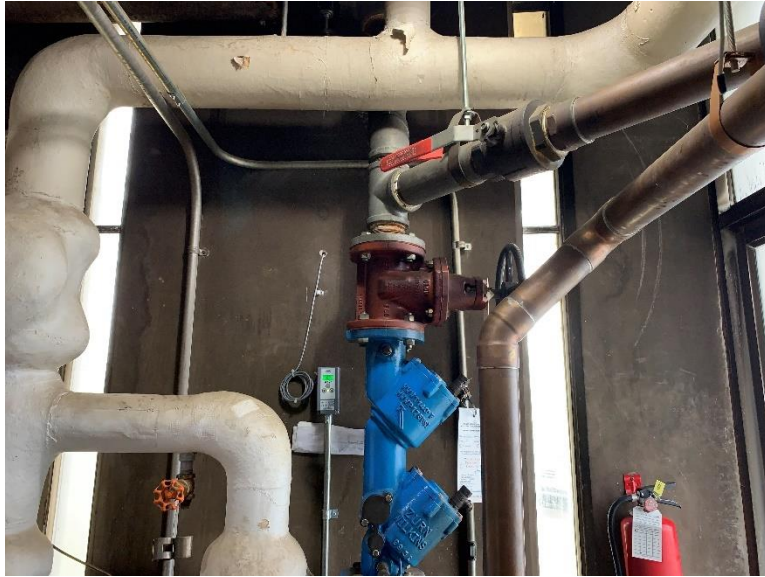
Photo 7: Domestic service water entrance
