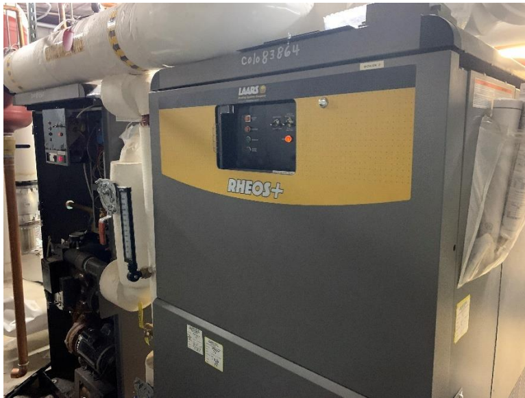
Photo 60: 2009 condensing boiler replacement
