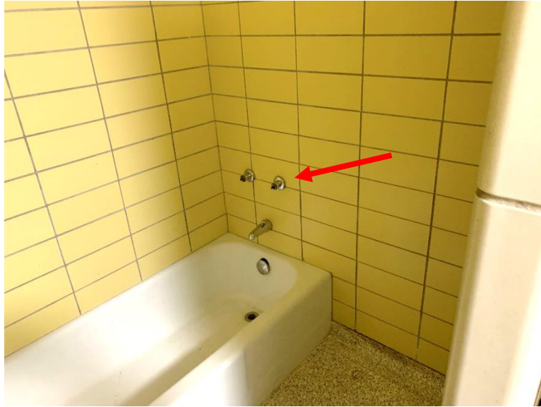
Photo 25: Existing bathtub with valve control removed?
