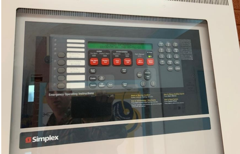
Photo 50: Huggins fire alarm system
