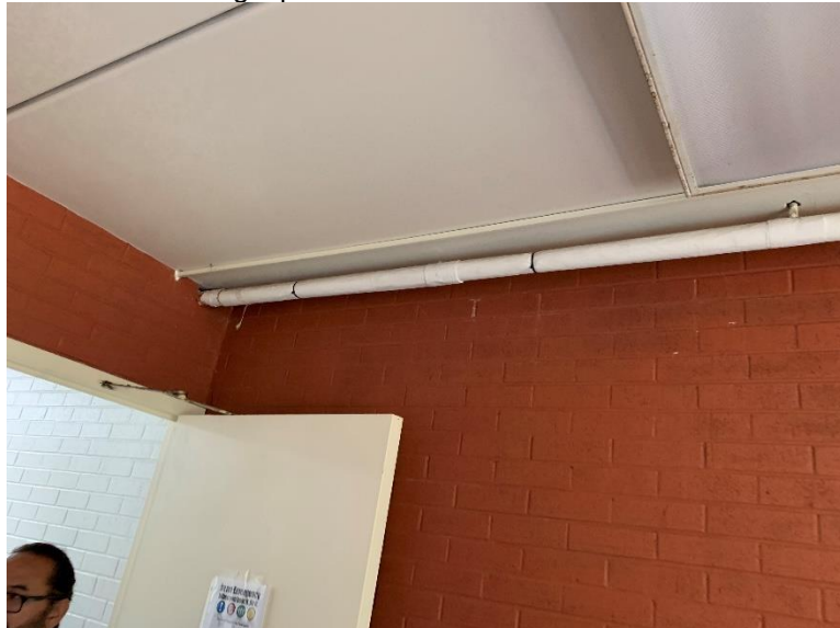
Photo 36: exposed piping in O'Connor dormitory entry
