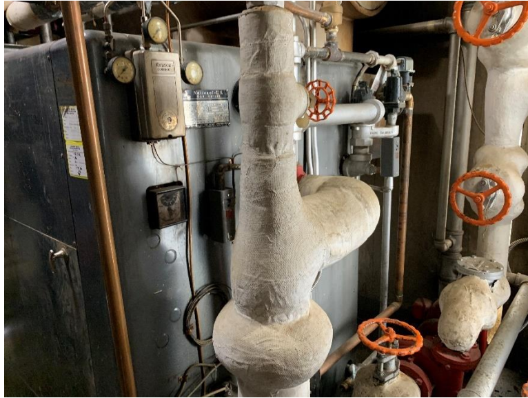
Photo 4: Existing gas-fired 3000 MBH hydronic boiler
