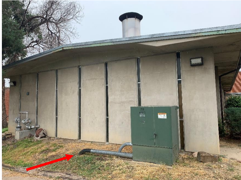
Photo 1: Student Center electric and gas utility services
