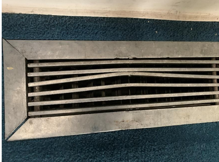
Photo 15: Existing damaged floor diffuser
