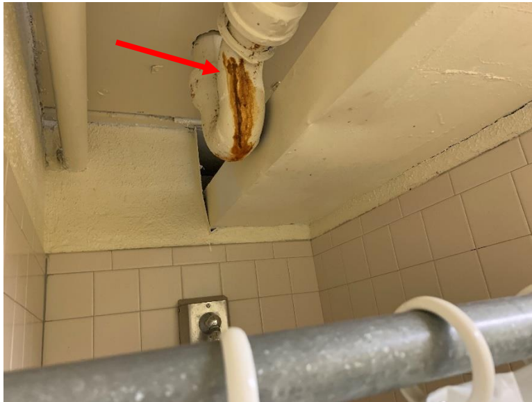
Photo 58: corrosion observed on exposed cast-iron sanitary trap
