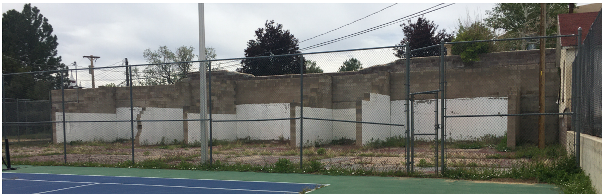
Figure E. View looking west to existing racquetball courts northwest of O'Connor, that have not been in use, not been maintained. Source: Hall Architects.
