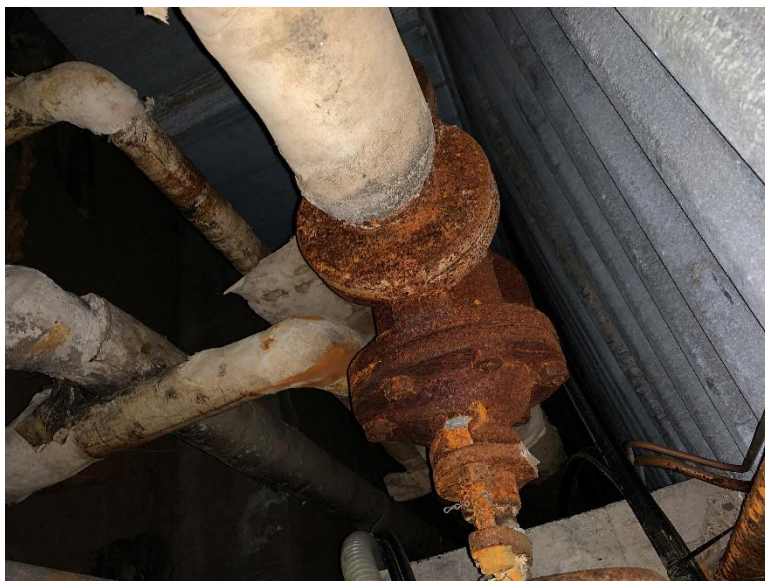
Photo 9: existing gate valve exhibiting extreme corrosion
