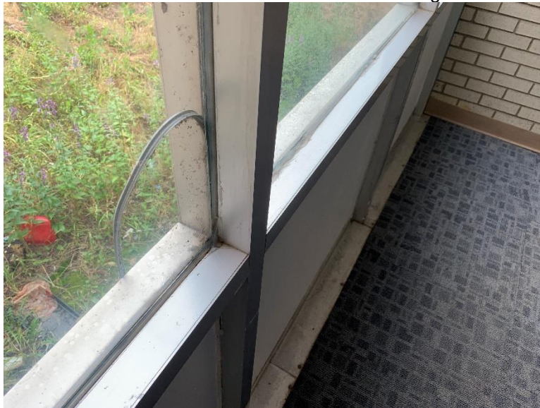
Photo 35: Single pane aluminum window with seal failure
