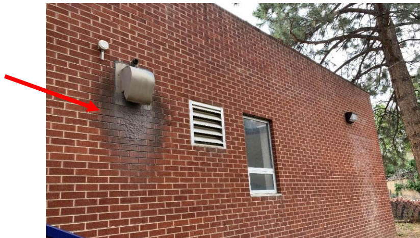
Photo 62: Lint accumulation at dryer vent
