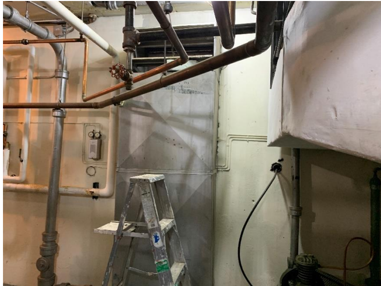
Photo 44: O'Connor combustion air ductwork
