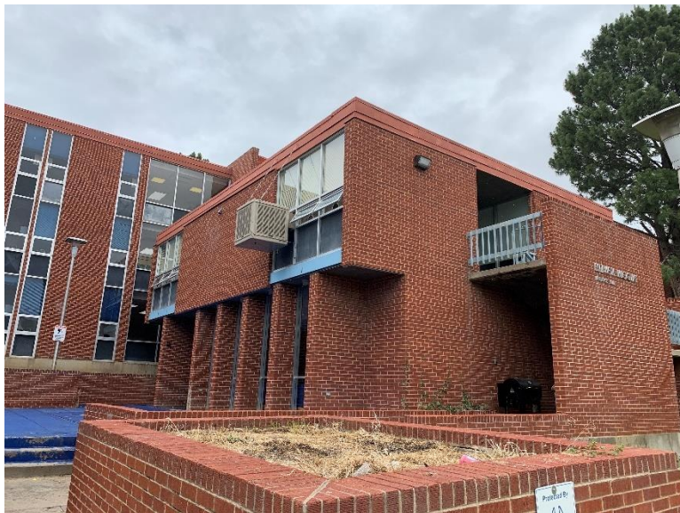
Photo 56: Huggins Hall resident apartment evaporative cooler
