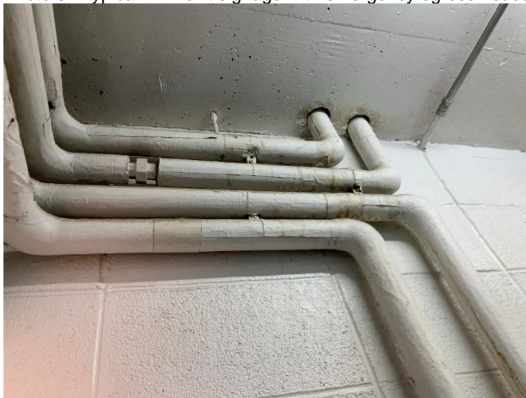
Photo 53: Suspect hard-cast ACM insulation elbows
