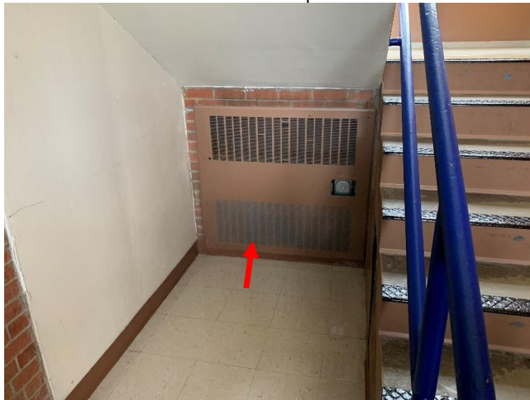
Photo 20: Johnson stairwell convection heater
