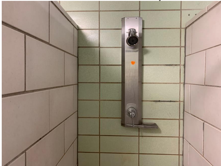
Photo 32: Romero Dorm institutional type shower fixture with SS concealed pipe cover
