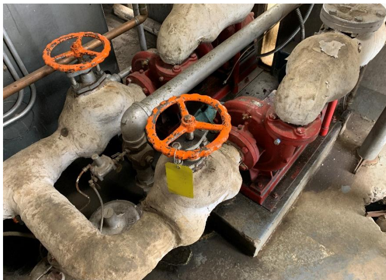
Photo 6: HW distribution pumps
