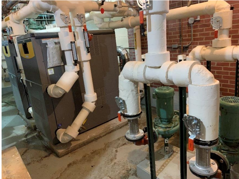
Photo 39: O'Connor boilers manufactured in August 2009 per nameplate
