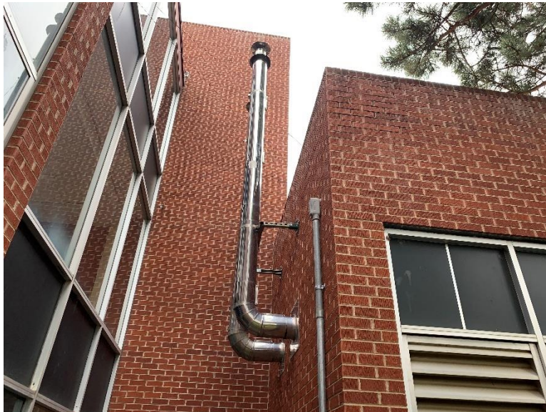
Photo 61: Category 4 A129-4C stainless steel boiler vents
