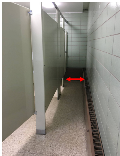
Figure J. Width of a standard aisle in a public bathroom measures 19" with convector. Current code minimum is 36". Source: Hall Architects
