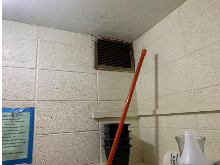
Photo 28: Johnson Residence Hall janitor closet exhaust
